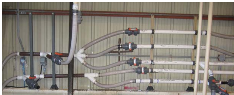
Figure 2 -Resin Transfer Manifold
