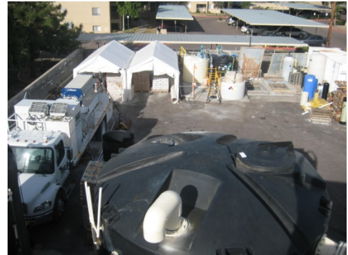
Figure 5 – The ZLD Facility
