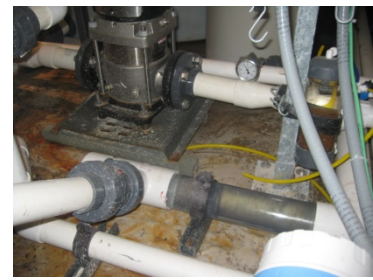
Figure 4 – Filtered BW Water
